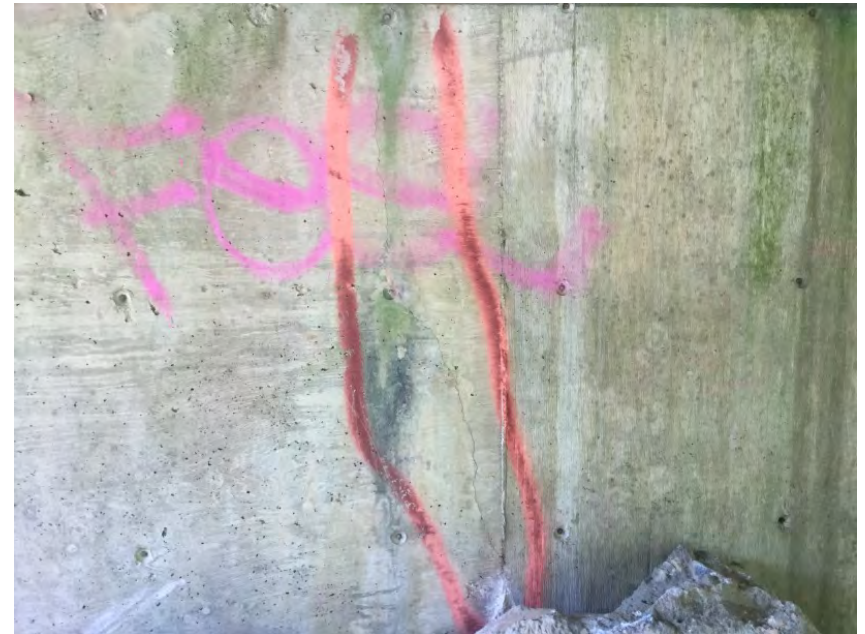
Hairline crack noted on left CIP
