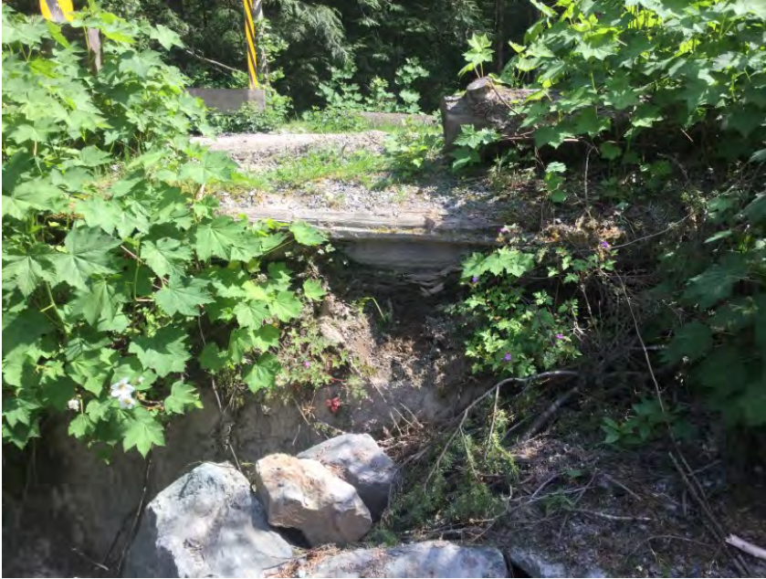
Logs retaining fill at either approach rotting
