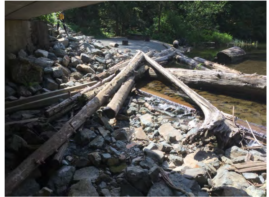
Debris at inlet to be removed
